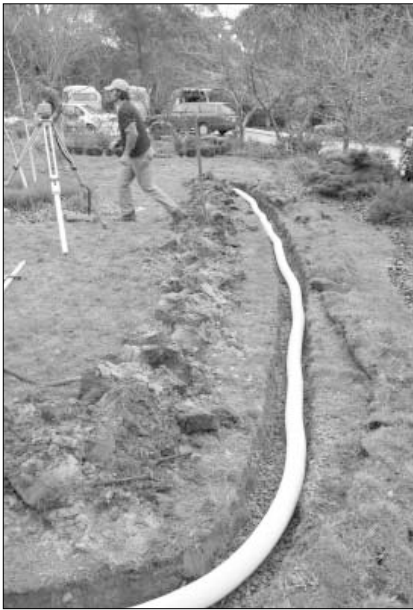
Laying of agricultural pipes in gravel filled trenches is one way to irrigate your garden with greywater.
